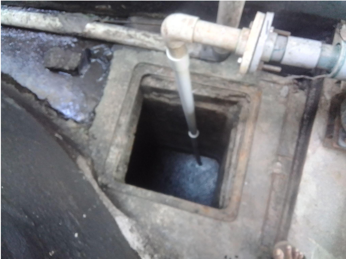
The entry point for climbing inside the filter feed tank of the STP
